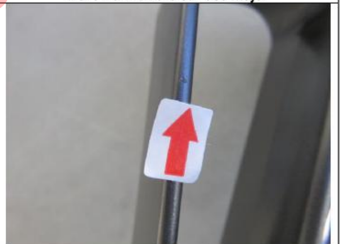
Dent mark on the surface-major
